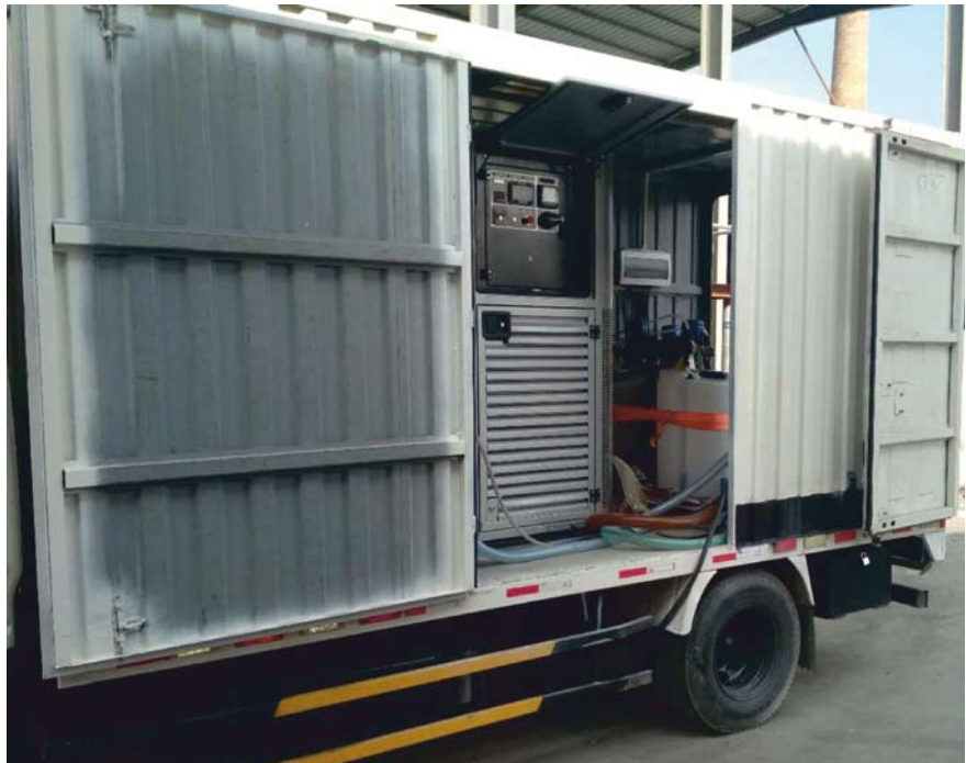
Commissioning of an AVS-150 System in a Paper Mill Wastewater Purification Line in China
